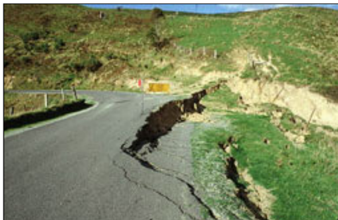
Figure A1: A landslide that has destroyed a road in the Corangamite region Photograph: A. Miner 2006
