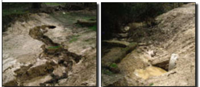
Figure A4: The start of an active gully erosion site, which washed sediments into a tributary of the Leigh River
