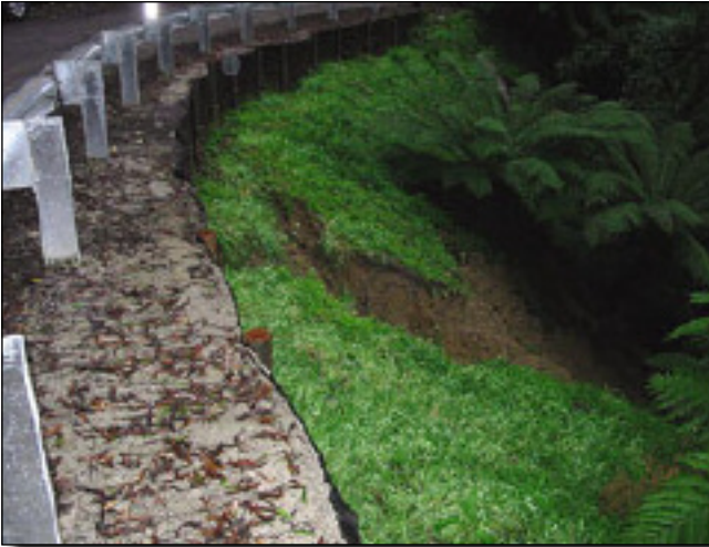
Figure D2: New failure below recent remedial works on Turtons Track (Gellibrand Landscape Zone) Photograph: A. Miner 2006
