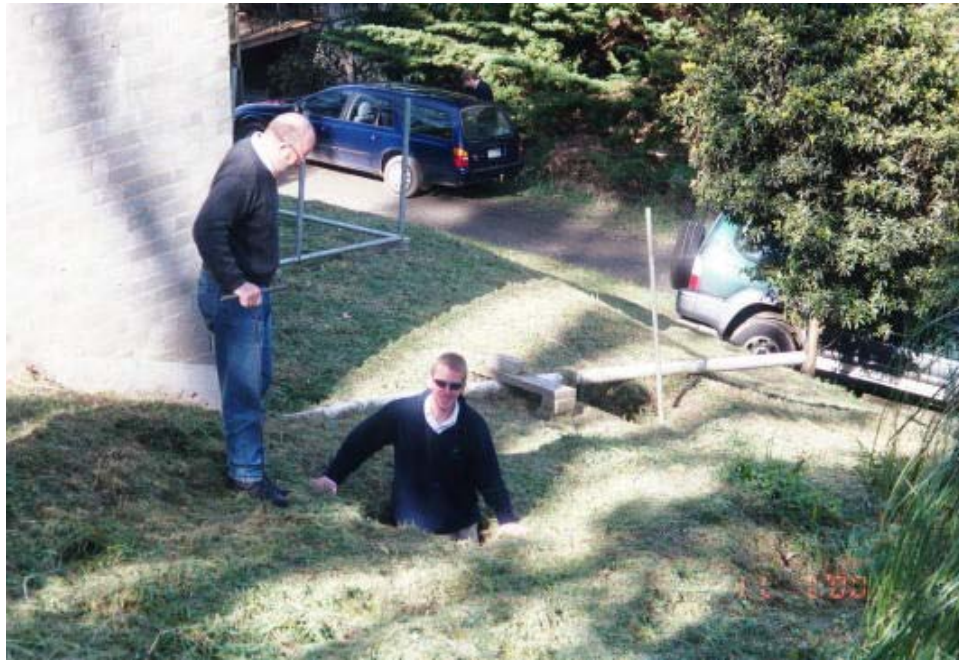
Figure B 9 Collapsed tunnel forming hole at the surface at Separation Creek.
