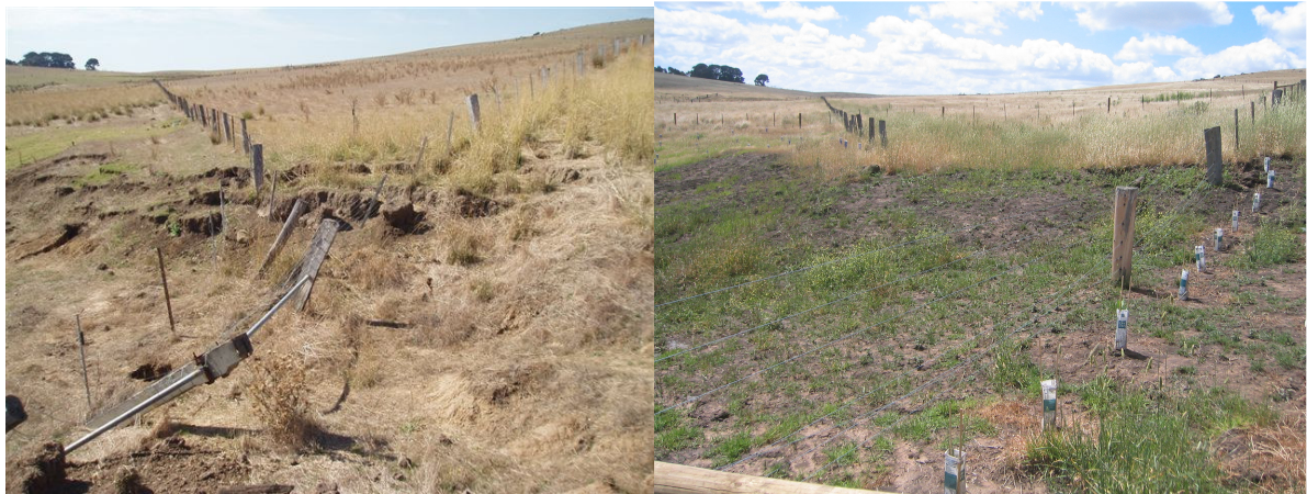
Photo set 2: Before and after photos of the landslide creeping under the boundary fence of the neighbours. After photo also one row of the tree belt planted along the new boundary fence to reduce sub-surface water entering the sensitive works area below. Photo taken looking south, south east.
