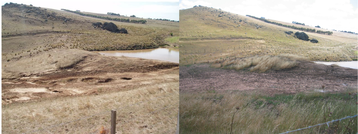
Photo set 1: Photo of tunnel erosion site before and after works, looking south east
