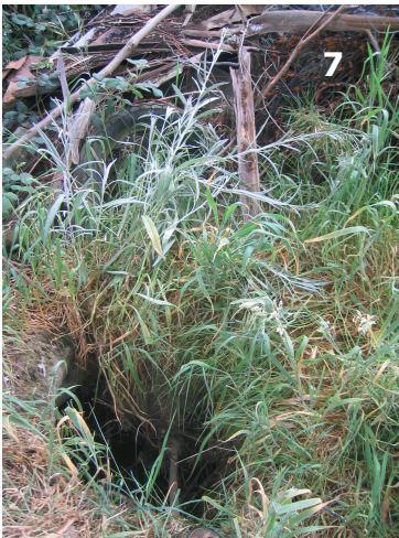
Photo 7: Tunnel which appeared after completion of works is still active. (same site as photo 5)
