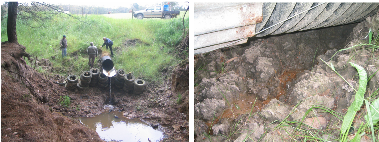
Photos 6 and 7: Further attempts at stabilisation of the overhanging pipe which has been undercut by erosion. Photo 7 shows the water leaking along the outside of the pipe causing the erosion around the pipe.
