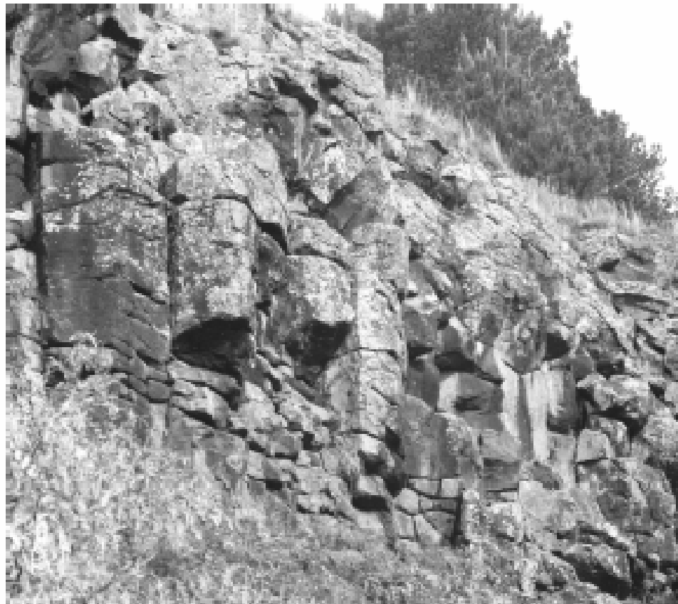
Figure 6. Undercut columns with open joints.
