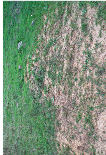
Figure 2: Partial collapse of tunnel with drying off lines visible.
