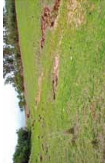
Figure 3: Tunnel collapse and surface clay deposits.
