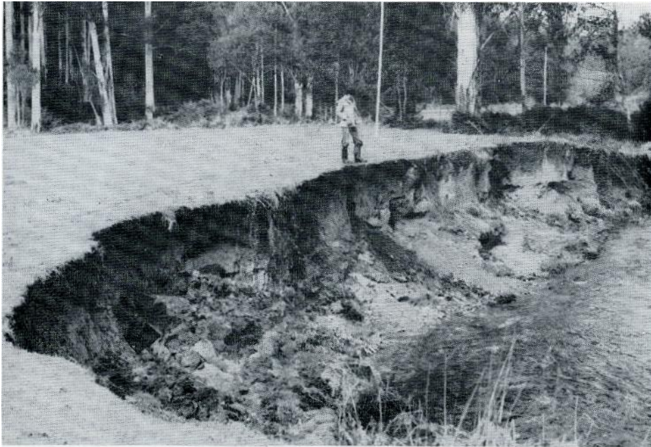
Plate 12. Active stream bank erosion along the West Tyers River. A loose stone embankment built to provide a summer swimming hole has directed flows on to the unprotected bank.
