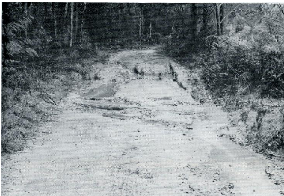
Plate 14. Tyers Junction sub-unit. Road through small drainage line. Regularly used tracks require regular maintenance. A blocked culvert may render tracks impassable.
