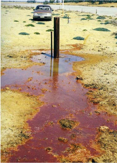
Figure 7.19 - This artesian bore, situated on the edge of the main Raak salina, monitors an interval at about 50 m in the Parilla Sand aquifer. Water seeping from a join in the PVC casing has deposited a coating of iron oxide over the casing and on the sides of a drainage ditch. The salina floor is heavily ferruginized, and islands in the distance have an ironstone base, which can be seen in Figure 7.20.
